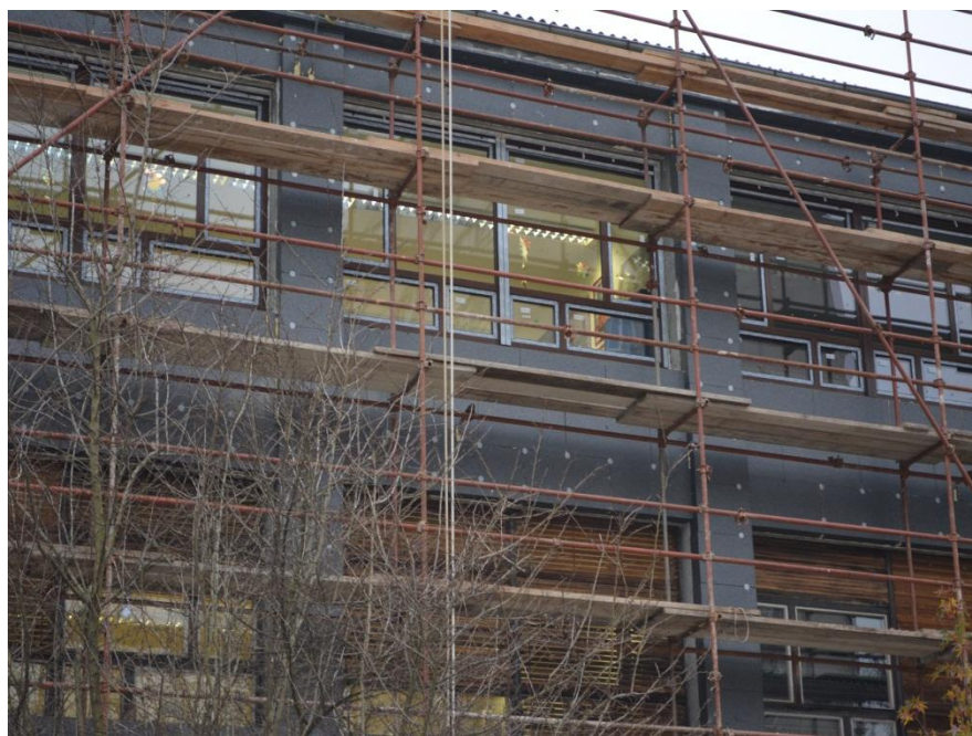
1. Thermal insulation of the external walls with the ETICS system made of a panels (expanded polystyrene) 18cm;
