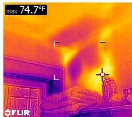
Missing Insulation – Summer Day E6 with MSX
