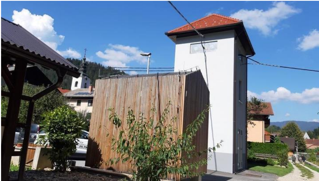
Image 28: System battery in Luče, Source: Borut Hočevar
