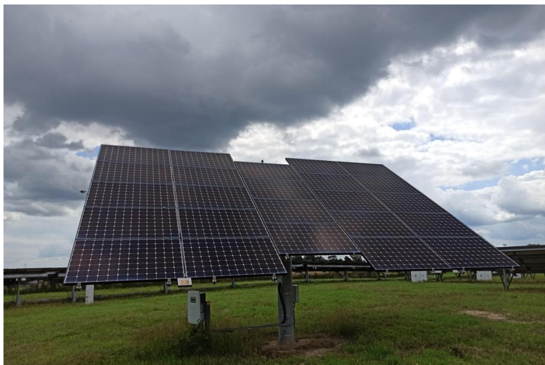
Image 20: Photovoltaic power plant in Marianka, Source: oze-invest.pl
