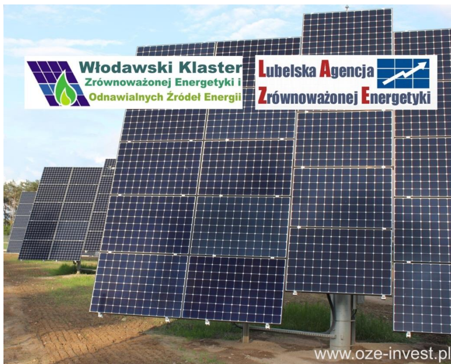
Image 22: Photovoltaic power plant in Marianka, Source: oze-invest.pl
