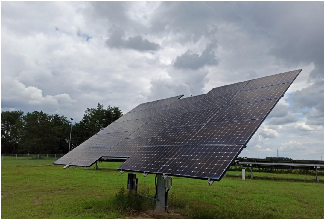
Image 21: Photovoltaic power plant in Marianka, Source: oze-invest.pl
