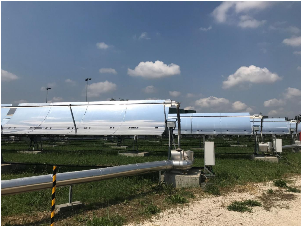
Image 15: Solar thermal power station near Forlì, Source: FMI
