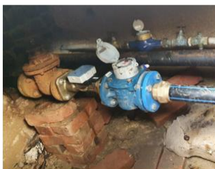
Water meters installed (implementation)
