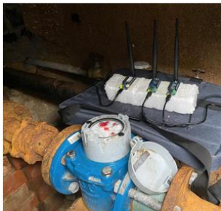
On-site measurements (planning)
