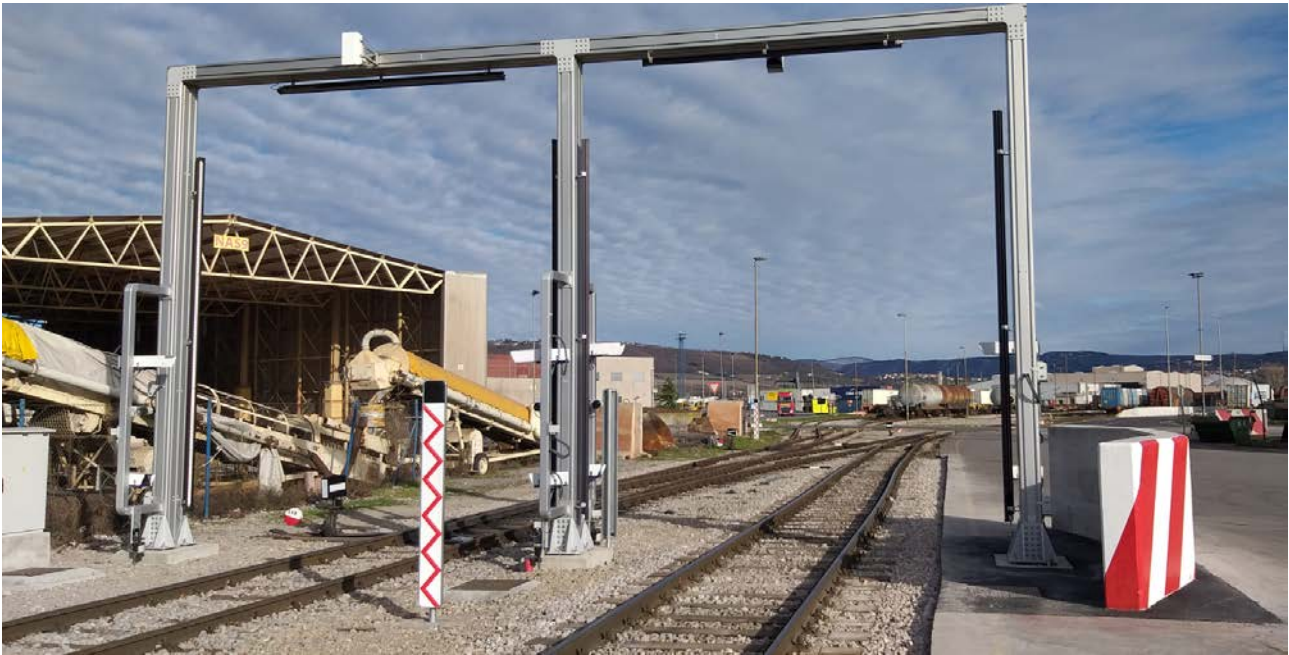
Figure 3: installed OCR system in the port of Koper (Source: Luka Koper's archive)
