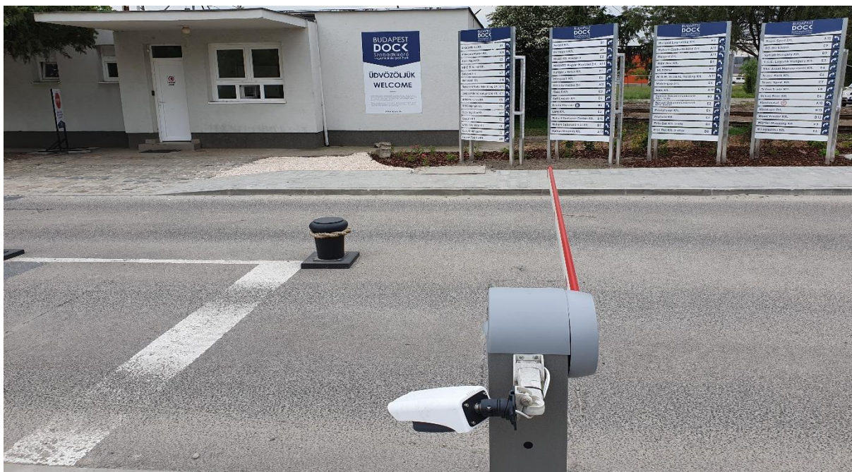
3. Image- Current access control system installed at BFL by Digital Entry System Control.
