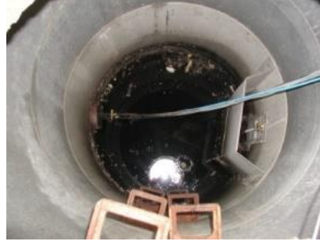
Rainwater sewer with switch diversion
