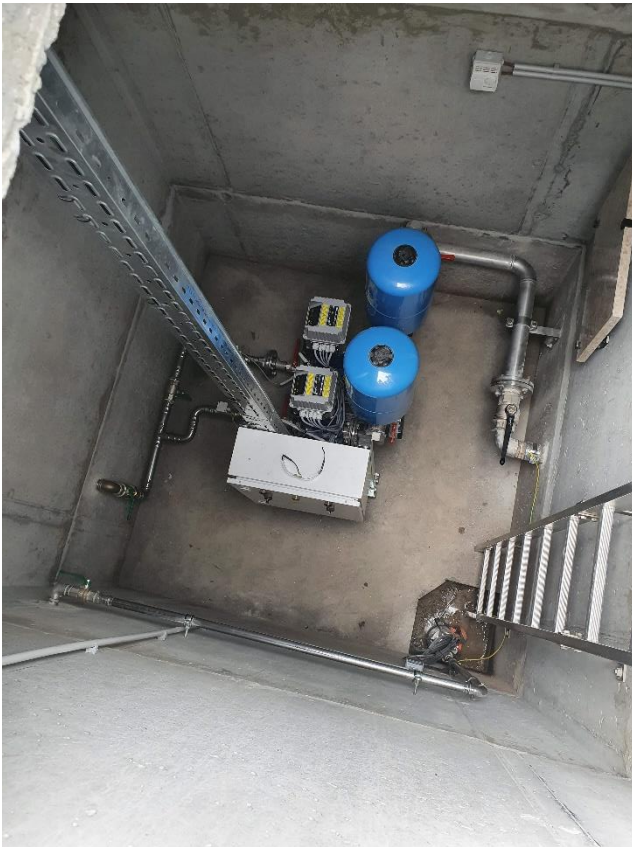
Figure 3: Pumps and electrical cabinet with automatics inside the shaft
