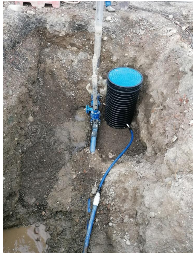
Figure 4: Connection points for rainwater and purified wastewater (hydrant) and drinking water (PVC shaft)
