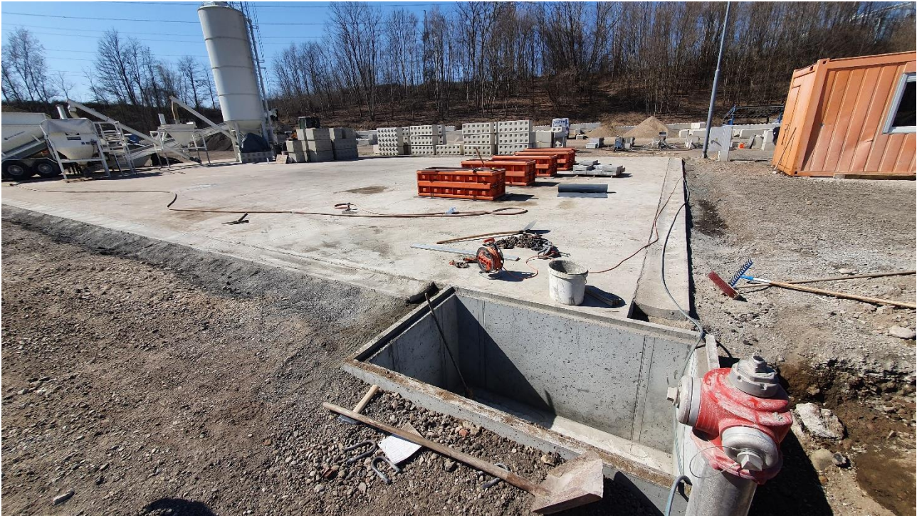
Figure 6: Drainage and the collection shaft for collection of rainwater mixed with discharged industrial wastewater from construction (during construction)
