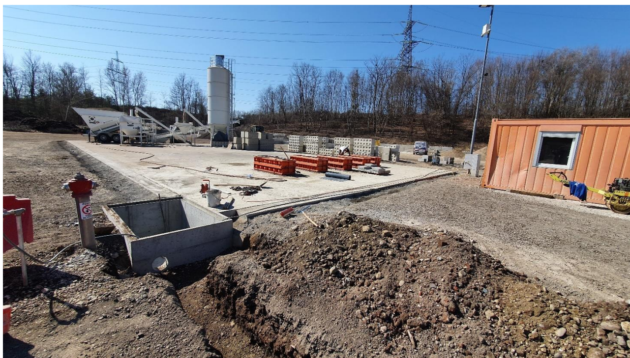
Figure 7: Hydrant with a "non-potable water" sign while "rainwater mixed with discharged industrial wastewater from construction" drainage and collection area is being built
