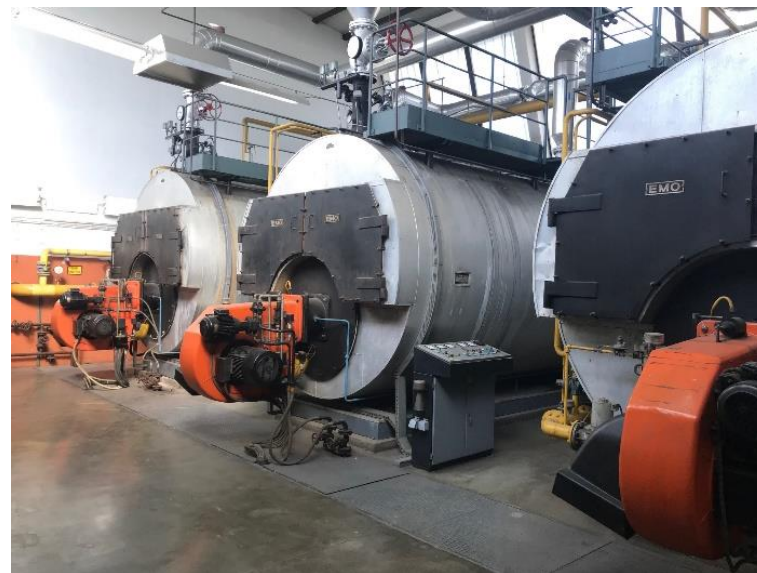
Existing boiler plant
