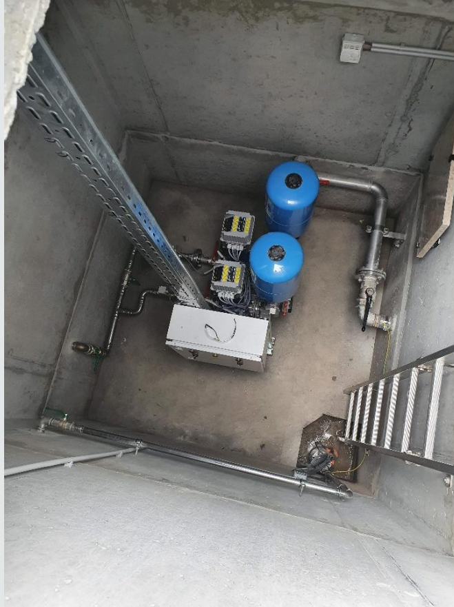
Figure 2: Hydro-booster station with two pumps inside the shaft
