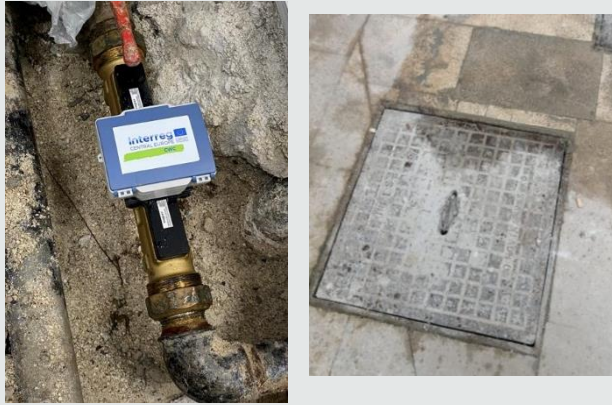
Water meter installed
