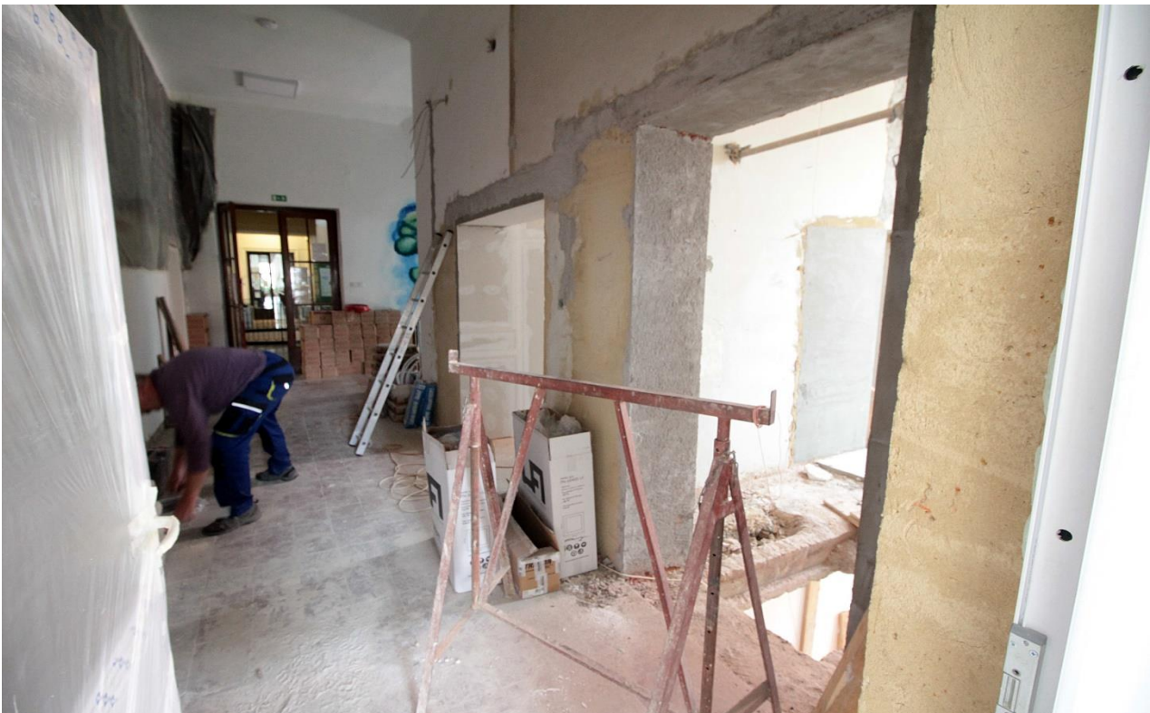
Fig. 3: Second floor east-wing of the building where the building activities take part
