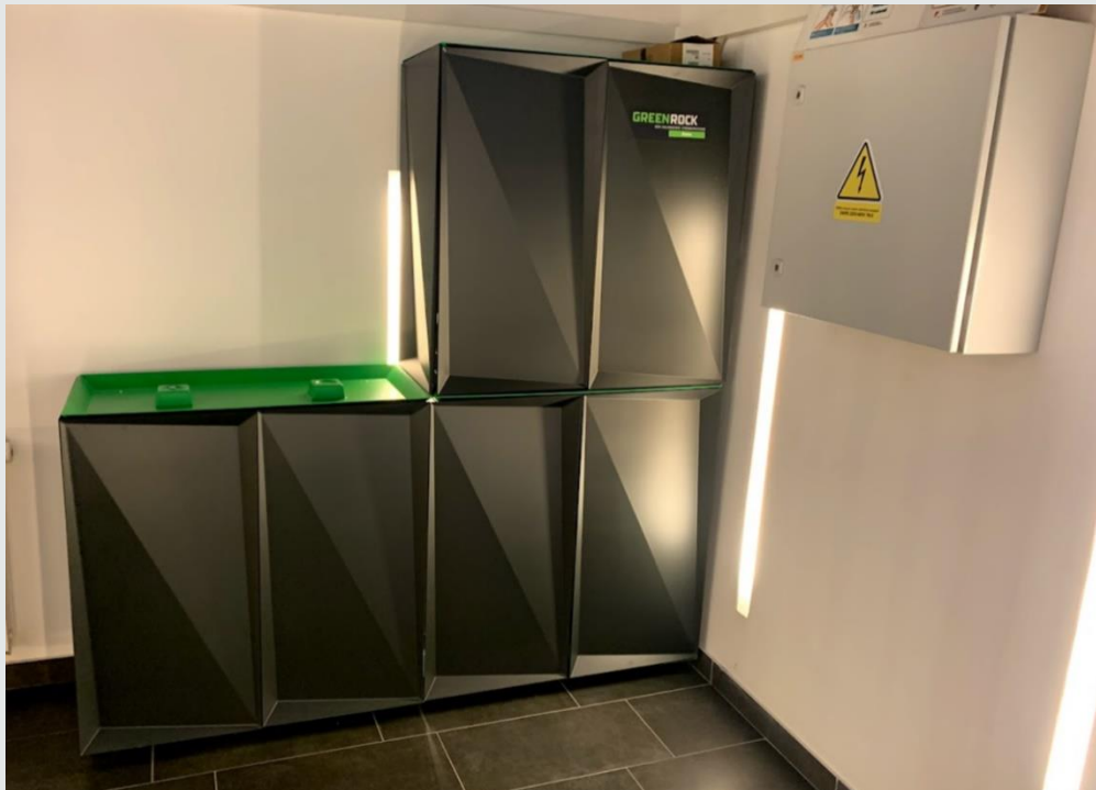
Figure 4: The storage (battery system) is placed in the premises of the Bračak Manor, in the basement next to the stairs. Source: REGEA 2021.
