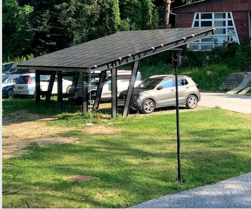
Figure 3: Installed photovoltaic modules Source: REGEA 2021.
