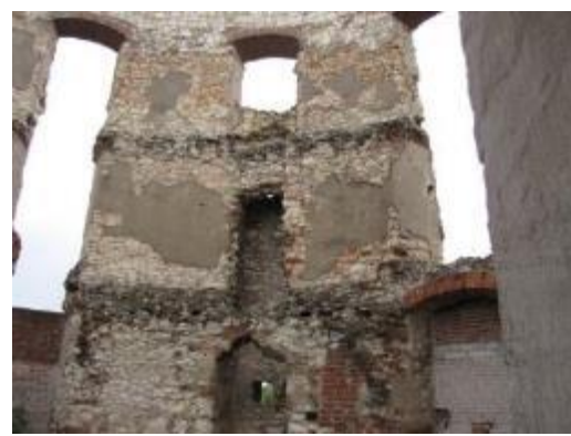
Photo 101 Plaster on the grand bastion provided with no protection
