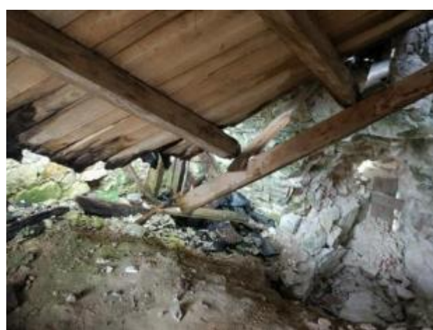
Photo 89 Damaged roofing which covers the basement of the south suite of rooms
