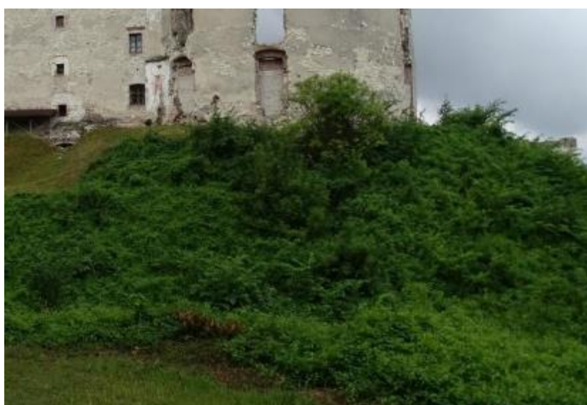
Photo 128 Bush growing in the moat.
