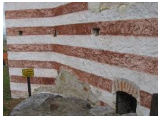
Photo 99 Gate house: plaster scaling
