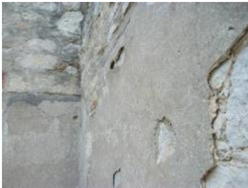
Photo 102 South suite of rooms: condition of the plaster
