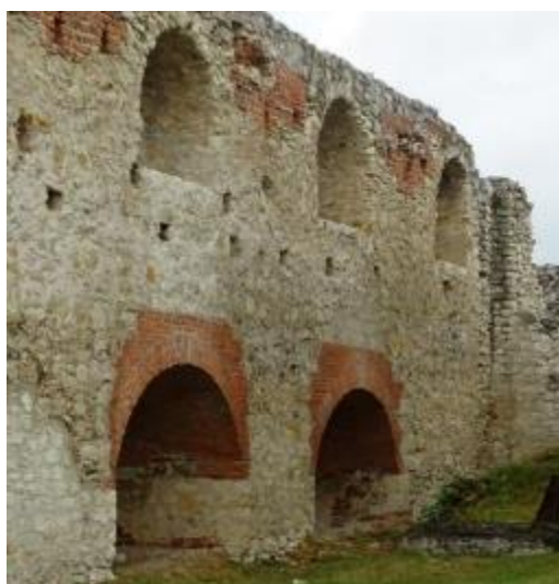
Photo 62 The north wall: repairing the face of the walls from the inside of the building
