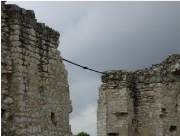
Photo 38 Tie beam connecting walls in the northern part of the premises - changing the static scheme
