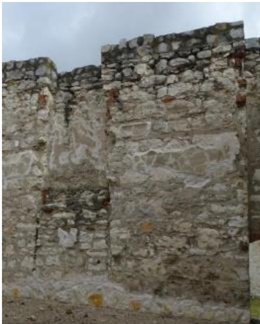
Photo 70 South suite of rooms - the face of the walls and plaster are considerably damaged where the original part of the wall conjoins the calcite coping.
