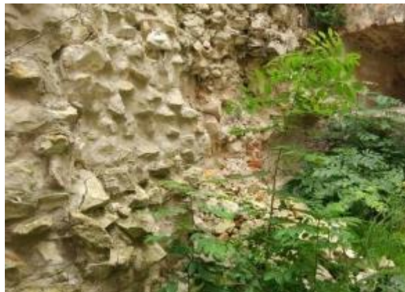
Photo 65 The wall of the Grand Bastion - north-east part of the castle Damaged part of the wall which was already a subject of preservation works.
