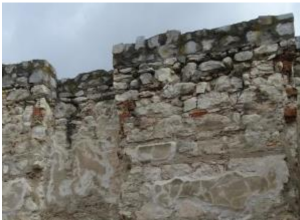
Photo 72 Wall coping protection - a new layer of foreign material added to the existing masonry
