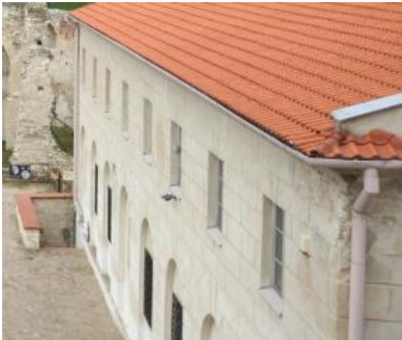
Photo 80 Leaky elements of the drainage system result in the corner of the building being damaged.
