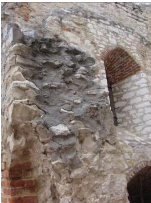
Photo 66 The wall of the Grand Bastion - north-east part of the castle Cement-based mortar used for repairing the falling-off face of the wall.
