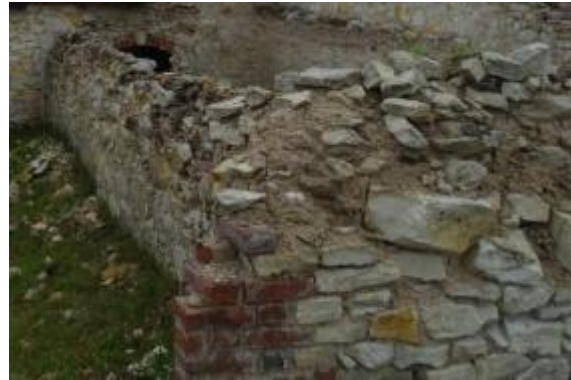
Photo 69 South suite of rooms - damaged grouts and stone and masonry material.
