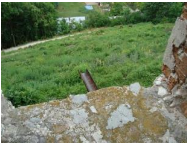
Photo 87 Gargoyles conveying water away from the castle
