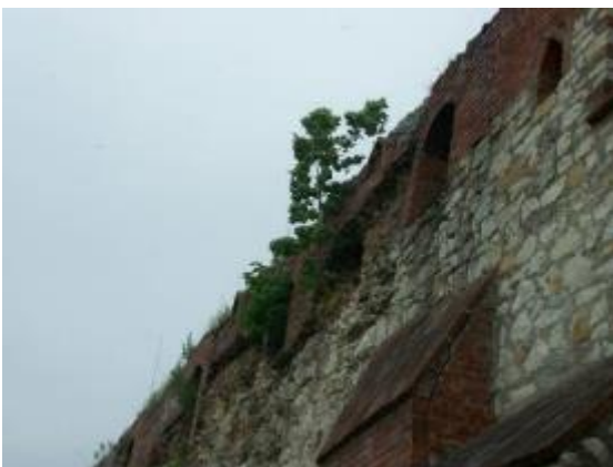
Photo 124 Young trees on the north wall coping
