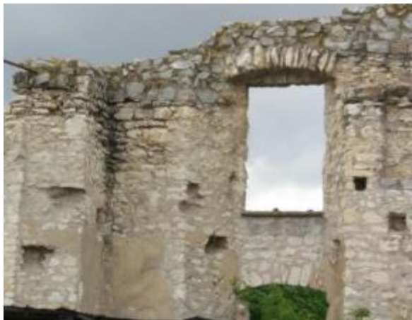
Photo 64 Wall of the Servants' building - north part of the castle. The repairs made in the lower parts are in satisfying condition. The face of the wall is degraded at the junction with the calcite crown.
