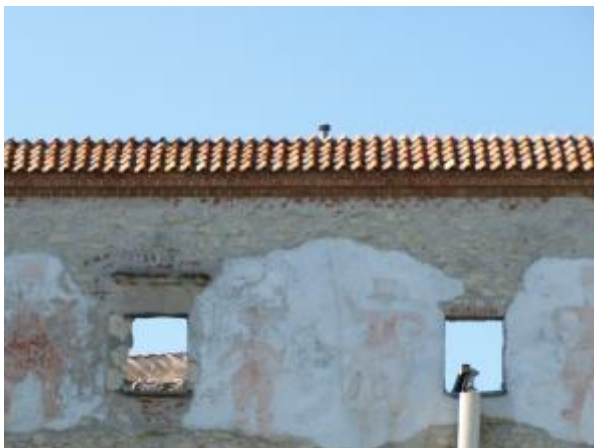
Photo 74 Wall coping protection - a new layer of foreign material added to the existing masonry; Ceramic roofing installed.
