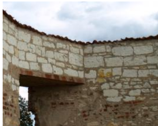
Photo 73 Wall coping protection - a new layer of native material added to the existing masonry; Ceramic roofing installed.
