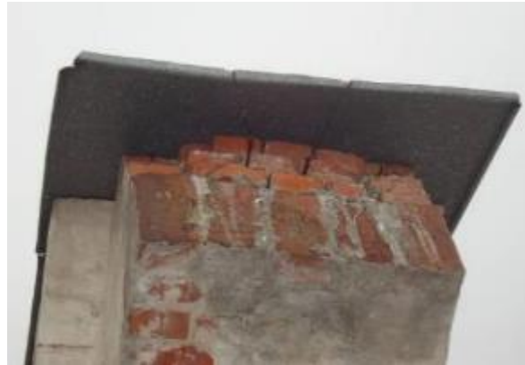
Photo 77 Wall coping protection: flat steel sheet
