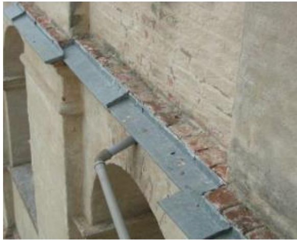
Photo 81 Metal elements fail to cover the cornice
