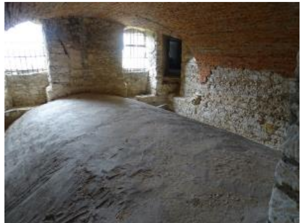
Photo 41 Laying concrete on non-original vaults with the purpose of improving their safe bearing capacity
