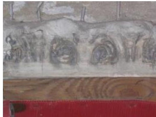
Photo 94 West apartment: moulding provided with wooden support
