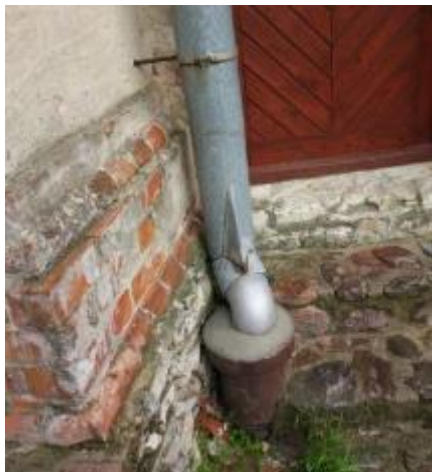
Photo 82 Outlet pipe connected to the storm drain system
