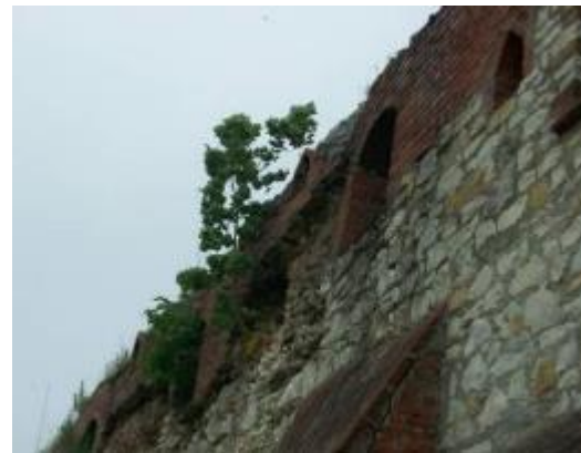
Photo 79 Adding a new layer of native material to the existing masonry; no roofing provided
