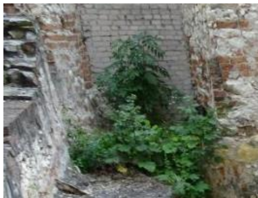
Photo 127 Plants on the projecting element of the east wing
