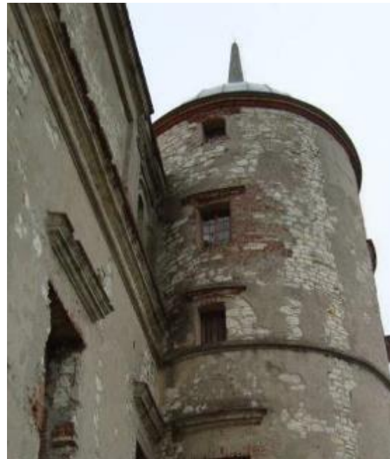
Photo 71 West tower - damp and defects on the face of the wall where the tower conjoins the west wing.
