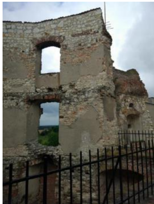
Photo 67 East tower Original parts of the walls are considerably damaged; the condition of the reconstructed upper part is satisfying.
